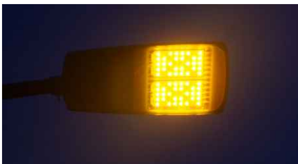
Figure 4.1.4. View of yellow LED street light and near-zero skyward flux emission. Photo: DGQACC. Government of Catalonia.
