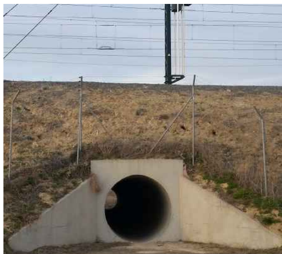
Figure 4.8.4. Burrows between fence and railway tracks. Although the fence is correctly installed around the culvert, gaps (see Figure 4.8.3) probably facilitated access by animals. Photo: Carlos Rodríguez.
