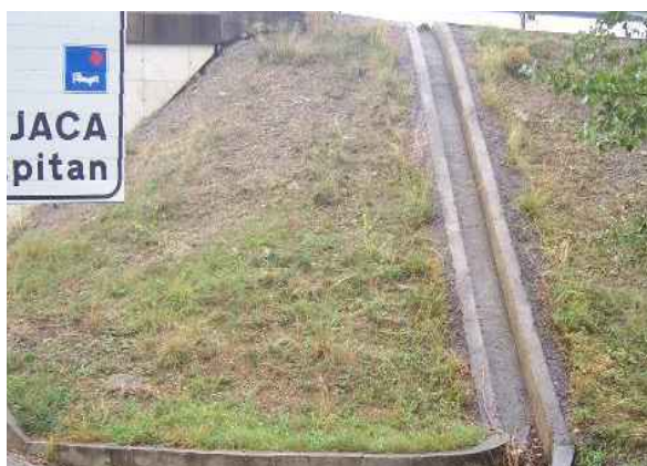
Figure 4.6.1. Run-off channelled by a gutter into a drainage system. Photo: Ministry of Public Works
