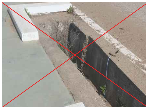
Figure 4.6.2. Culvert between two roads. A trap with no escape for small animals. Photo: Carlos Rodríguez.
