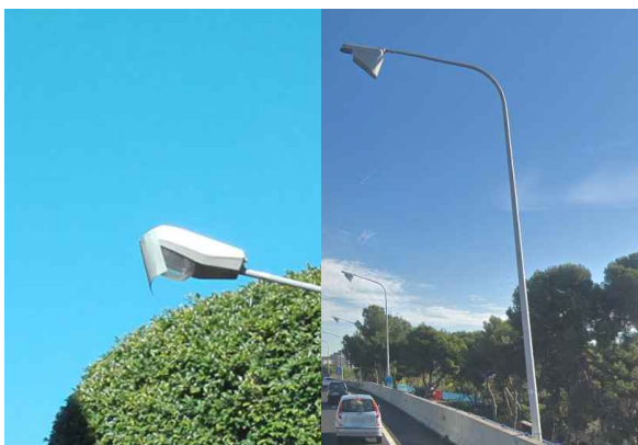
Figure 4.1.3. General and detailed view of shielding options on a Barcelona motorway. It avoids the intrusion of light in areas near the infrastructure. Photo: DGQACC. Generalitat de Catalunya.
