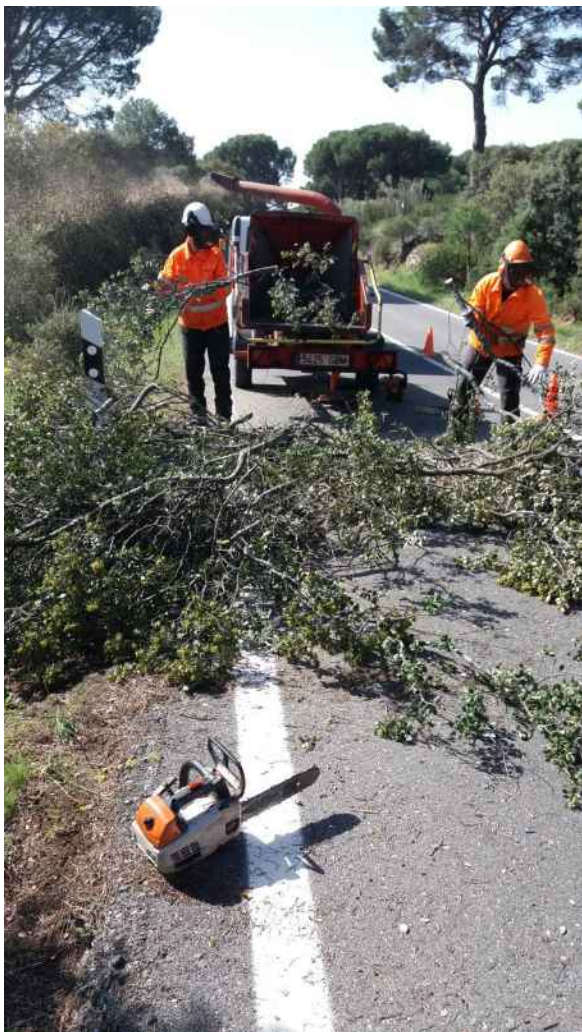
Figure 4.9.1. Manual verge clearance in a forest zone to reduce the presence of fauna in its immediate surroundings and increase their detection at a distance by drivers, thus reducing the likelihood of collisions. Photo: Community of Madrid.
