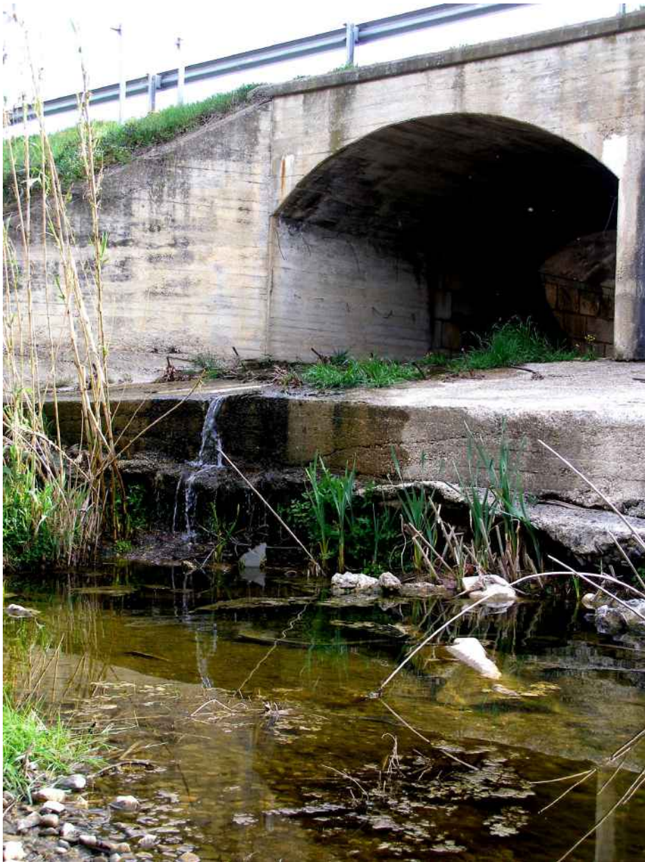
Figure 3.8. Bridge over the Burgantó River (Girona). The differential erosion on the concrete bed and the natural watercourse downstream from the bridge forms a barrier to the movement of aquatic animals along the river. Photo: Miguel Clavero.
