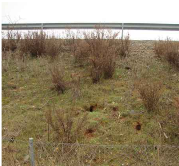
Figure 4.8.1. Rabbit burrows on motorway embankment Photo: Government of Navarra.
